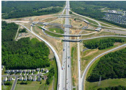
STV Incorporated's "I-485 / I-85 "Turbine" Interchange in Charlotte.
